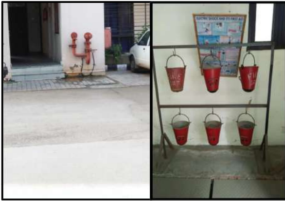
Fire Fighting Equipment
